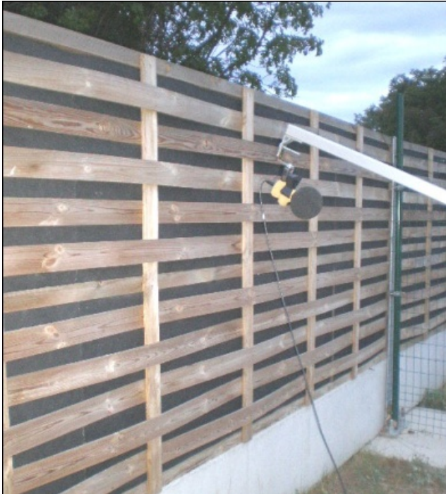
Figure 6. Barrier that doesn't meet minimum dimension requirements.
