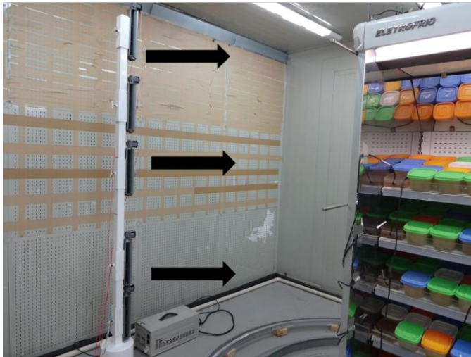
Fig. 3 Location of centrifugal fans used to provide auxiliary ventilation.
