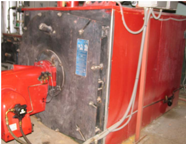
Fig. 3 Picture of the fully monitored facility
