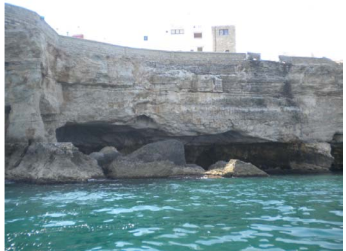
Fig. 7 mass movements: cave roof collapses (coastal sector V)
