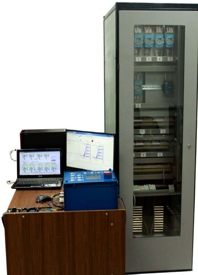
Fig. 5 mapping belt conveyor controlling hardware connected to the simulation model of whole mines factory
