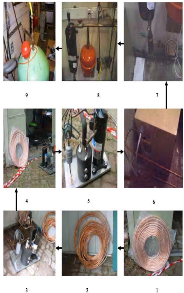
Fig. 4 Preparation of coils (1-2), installation of heat pump (3-6) and connection of water supply system (water pump, flow meter, expansion valve and the boiler) (7-9)
