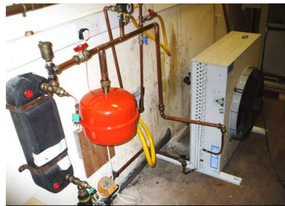
Fig. 15 The connections of the heat exchanger, water pump, heat rejection fan and expansion valve
