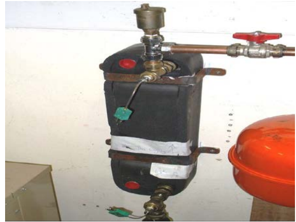
Fig. 14 The heat exchanger
