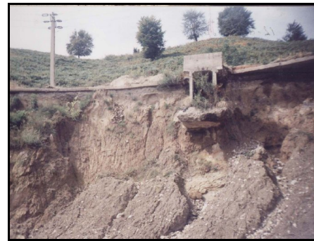
Fig. 16. Section of road affected by slip
