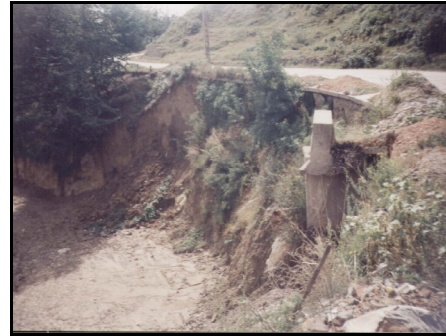
Fig. 17. Overview of the landslide slope affecting DC 29 road
