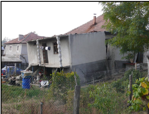
Fig. 14. Aspects of the lignite exploitation impact on building in Seciuri
