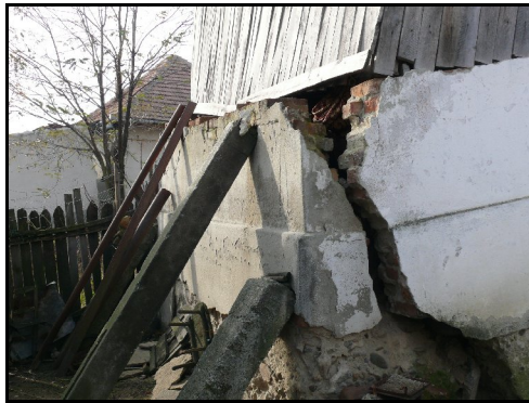
Fig. 13. Aspects that show how the buildings foundation was affected
