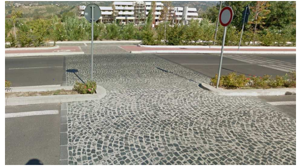
Fig. 6 Particular anomaly along the test site
