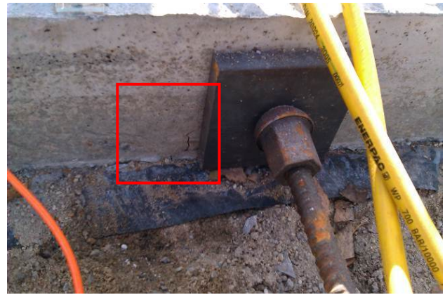
Fig. 12 Cracks near anchor of middle prestressing threadbar
