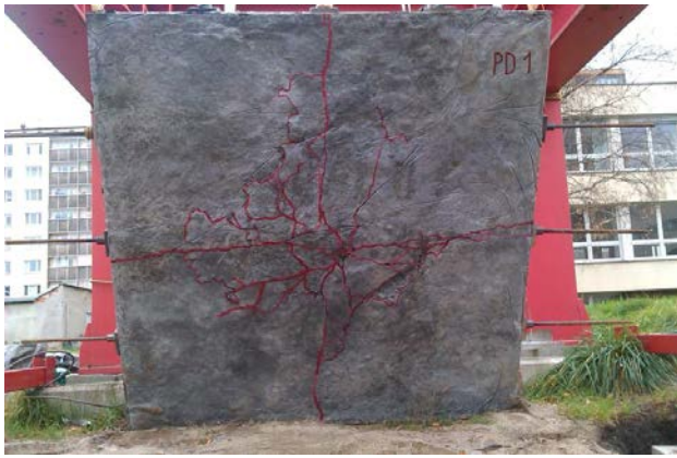
Fig. 15 Course of cracks on the contact surface of post-tensioned concrete industrial floor model
