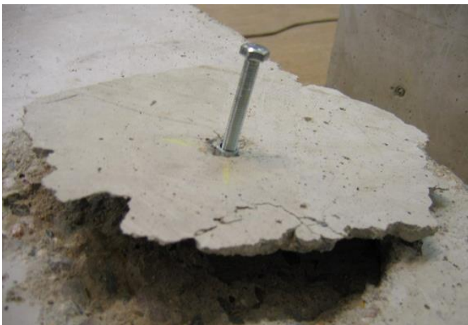
Fig. 14 failed specimen (concrete-cone failure)
