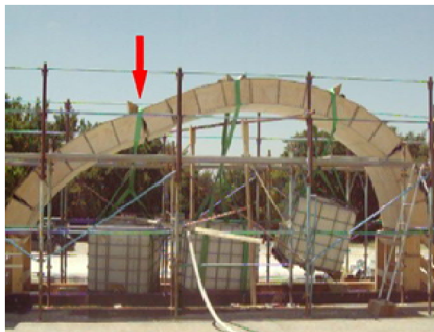
Fig. 11 collapse mechanism and achievement of the hinges in the arch with an asymmetric load condition
