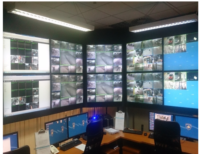
Fig. 1. Centre for borderline monitoring
