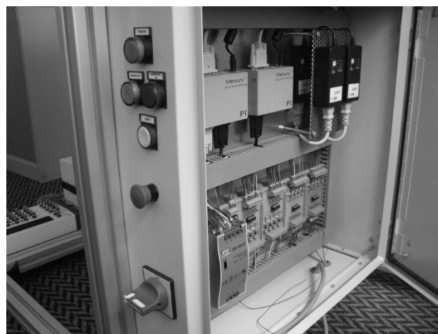
Fig. 1. Electrical control unit
