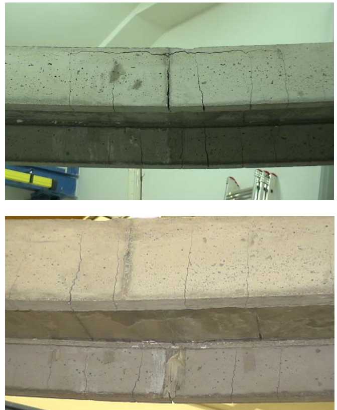
Fig. 12 Test specimen “D”: failure mechanism
