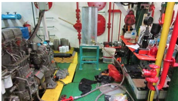
Fig. 6 Daily tank pipe to Main Engine (M/E)
