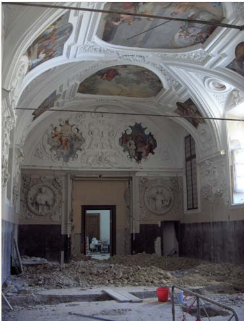
Fig. 6 - The Chapter Hall consolidated vault with the metallic tie-rods during the restoration works.
